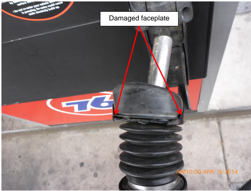
Photograph # 7: Damaged faceplate on nozzle # 3.
