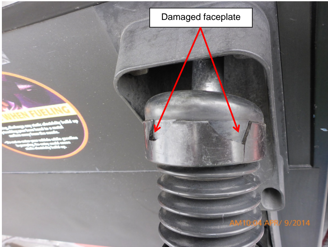
Photograph # 9: Damaged faceplate on nozzle # 6.
