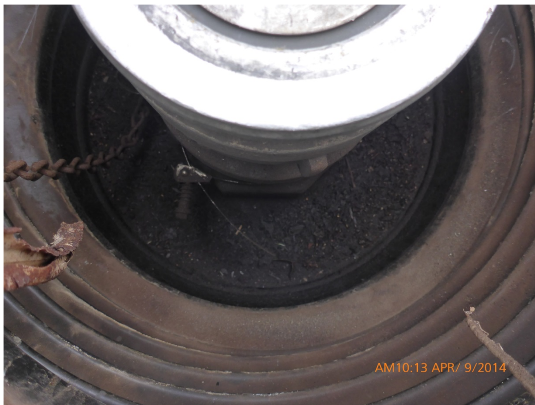
Photograph # 2: Debris in the vapor adaptor spill bucket of EU A02.
