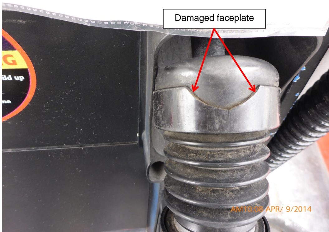
Photograph # 12: Damaged faceplate on nozzle # 9.
