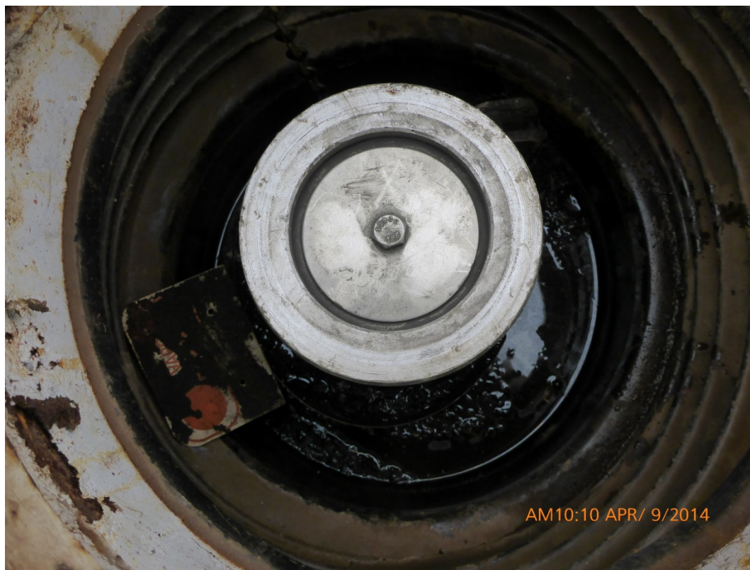
Photograph # 1: Liquid and debris in the vapor adaptor spill bucket of EU A01.
